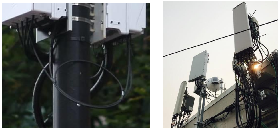
Typical poorly restrained looped cables
